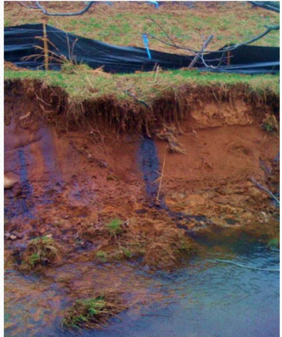
Drill site, Harrison County, WV. Landowner reported seeing oily substance bubbling up from ground and into stream. Driller later cited for putting a well pad on top of a wetland area.
