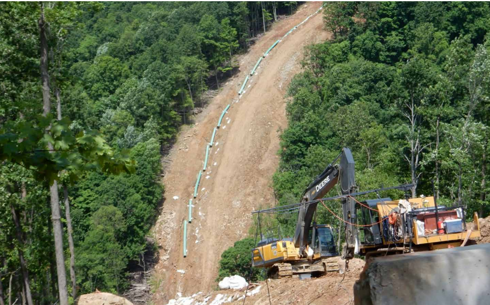
Above: Stringing out pipe and pipe being laid into the previously dug trench in WV. Photo by Bill Hughes, Ohio Valley Environmental Coalition, June 2016
