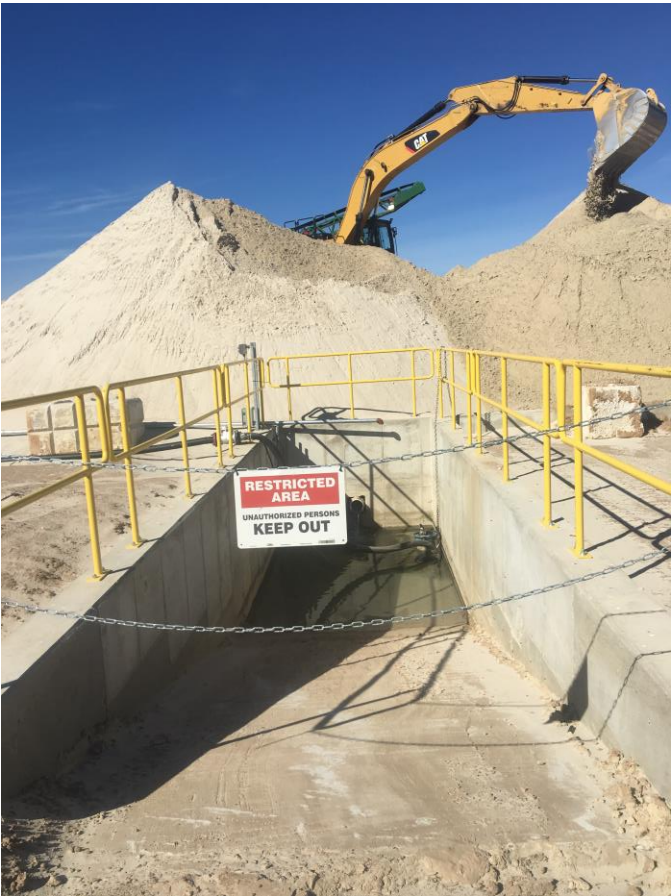
Photograph 6. Washed Sand Piled onto Drain Slab
